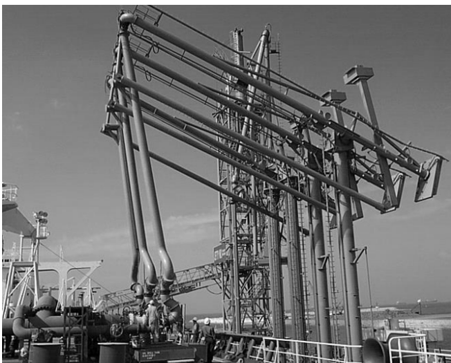
Figure 1. Loading arms for loading/unloading tankers in the oil terminal [6]
